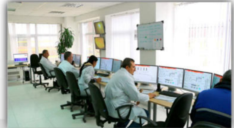
CCR - Central Control Room
