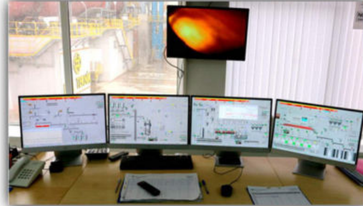
CCR - Central Control Room
